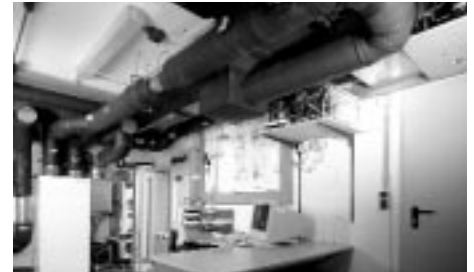
Fig. 1: Test stand for compact ventilation units in the Freiburg Solar House.
