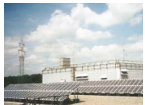
Fig. 6: "Karlsruher Sonnendach" with a rated power of 50 kW p .
