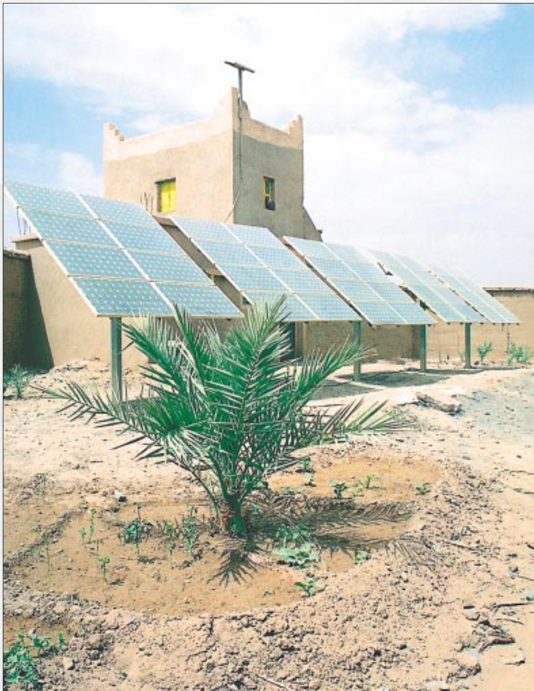
Photovoltaic pumping station for drinking water and irrigation in the village of Ifert, Morocco. Another photovoltaic array for the drinking water disinfection unit is mounted on the roof (see article on p. 78).
