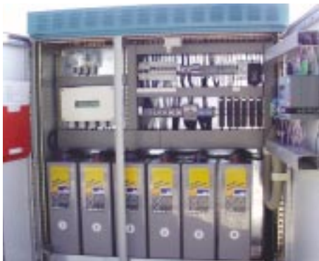
Fig. 3: Switch box to house the energy storage unit and control electronics. The heat exchanger to cool the batteries can be seen on the roof. It is powered with excess electricity from the photovoltaic generator.
